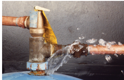
PHOTO A. A plastic-lined tank rusted through at the connection.
